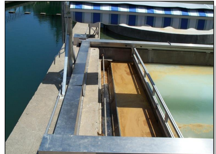
< Bangeojin Plant of Ulsan City(DAF) >
